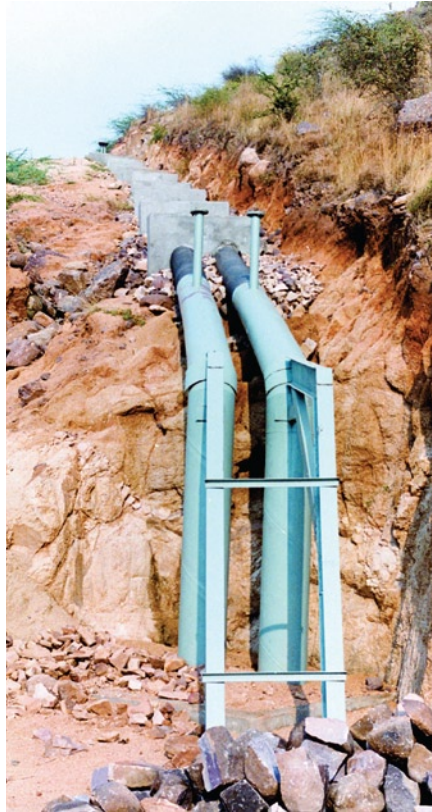
A pipeline becomes a lifeline
